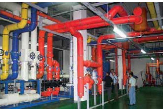
Customer substation in Cheongju, Korea
