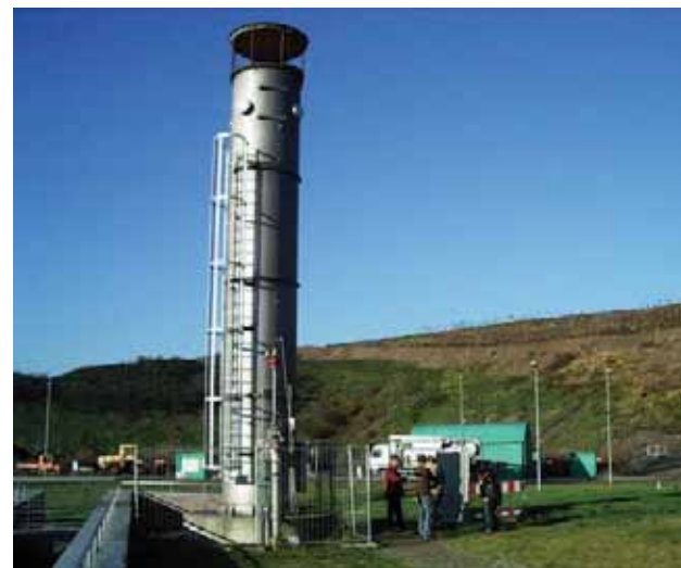
High temperature incineration flare for landfill gas
