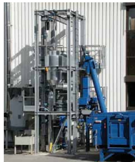
Fluidized bed gasification plant at Fraunhofer UMSICHT, Oberhausen
